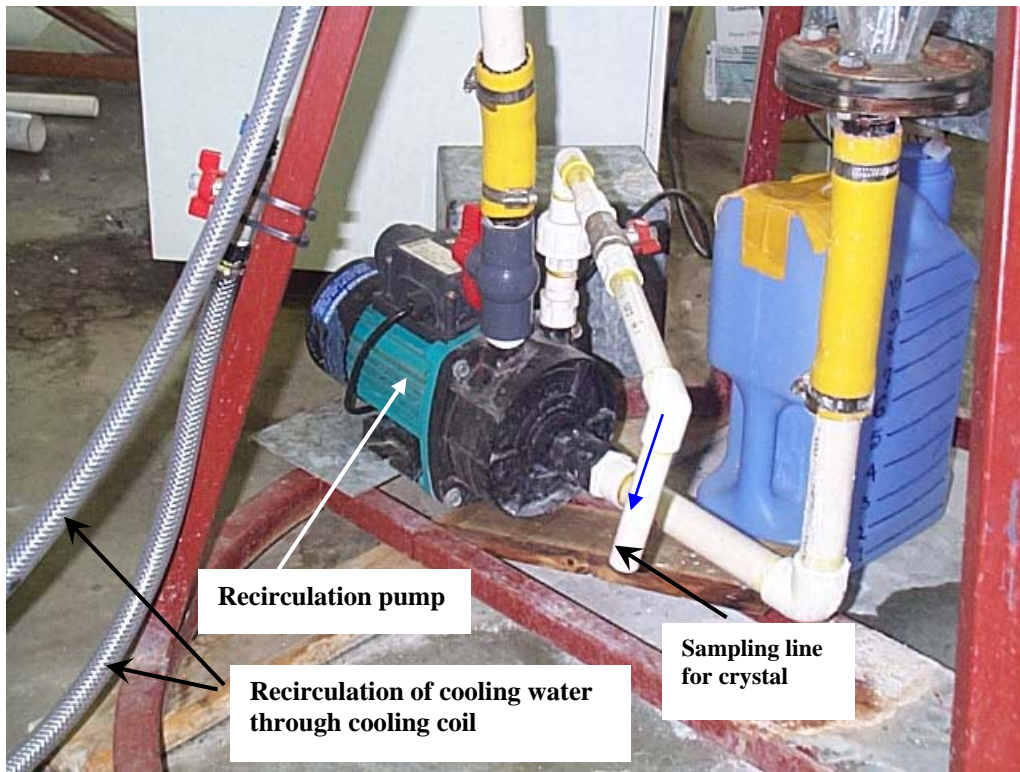
Figure 4.4 Sampling of struvite crystal through recirculation pump
