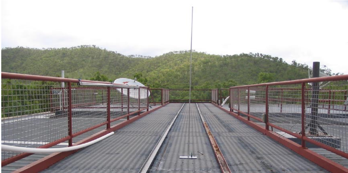
Figure 4-24: Prototype antenna installed on roof top
