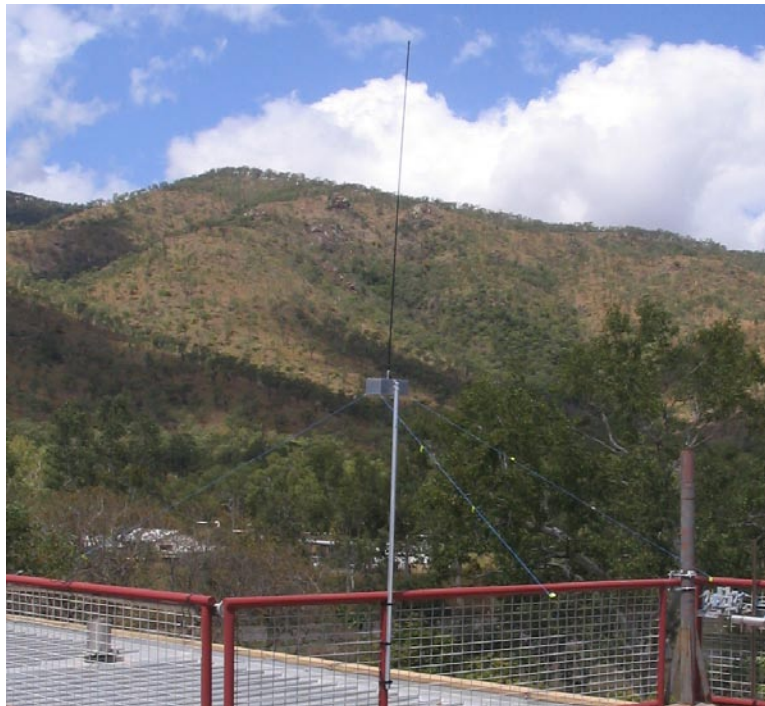
Figure 6-1: Transmitting node installed on roof
