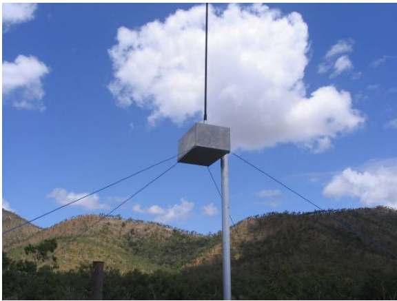
Figure 5. Node installed with radials
